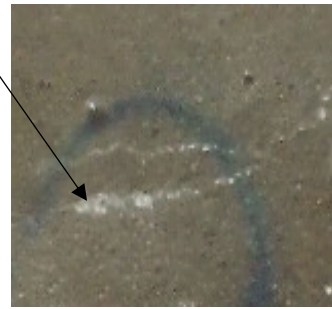
Plate II: Calcites in Cracks
